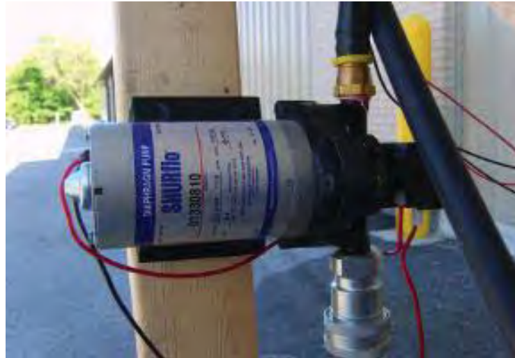
Figure 5.3: Water pump installation
