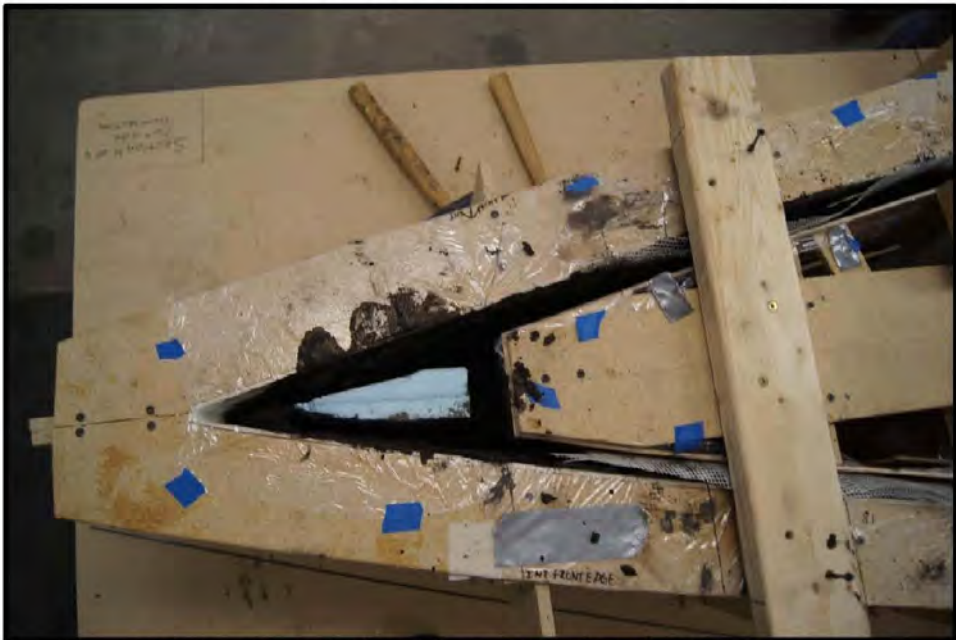
Figure 12: Placement of the solid foam wedge in the bow and stern, and top view of the 1" thickness obtained from attaching interior mold.
