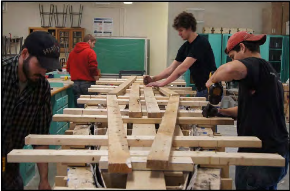
Figure 11: Installing the interior mold onto the exterior mold, then vibrating concrete down the sides to obtain the consistent 1" thickness.
